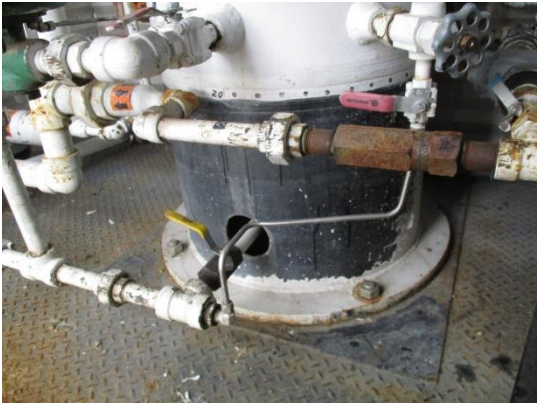
NO INSPECTION PORT IN SKIRT
